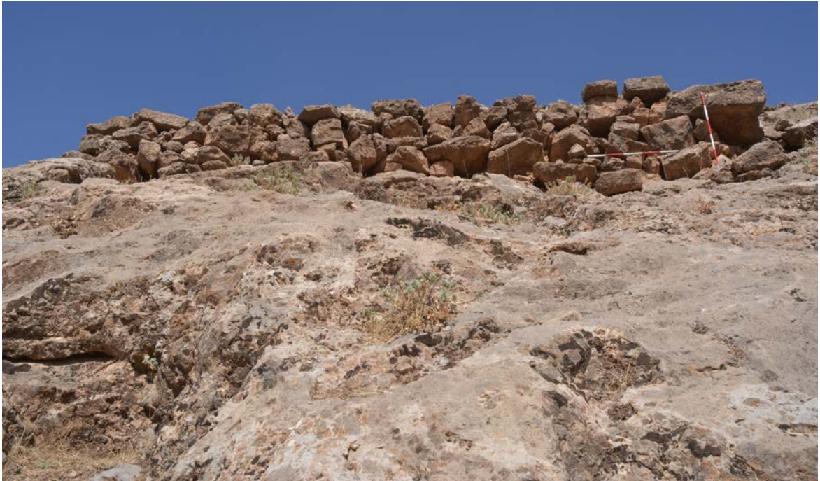
Fig. 12: Kapchigay – slope of Ketman Chapti. A part of the wall on the slope. Photo T. Votroubeková.
